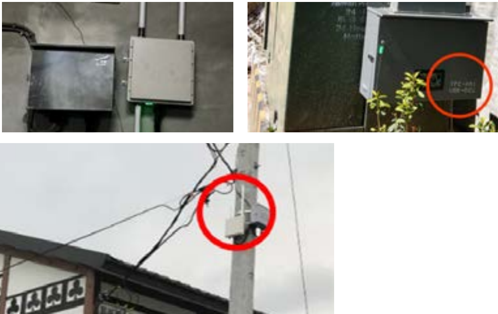
Figure 5: DCUs installed at three different locations in Taiwan. Ubiik provides 320 DCUs to provide communication that will provide service to roughly 280,000 FAN devices in Taiwan by the end of 2020. Middle location is a pole mounted DCU, while right location is mounted at ground level.
